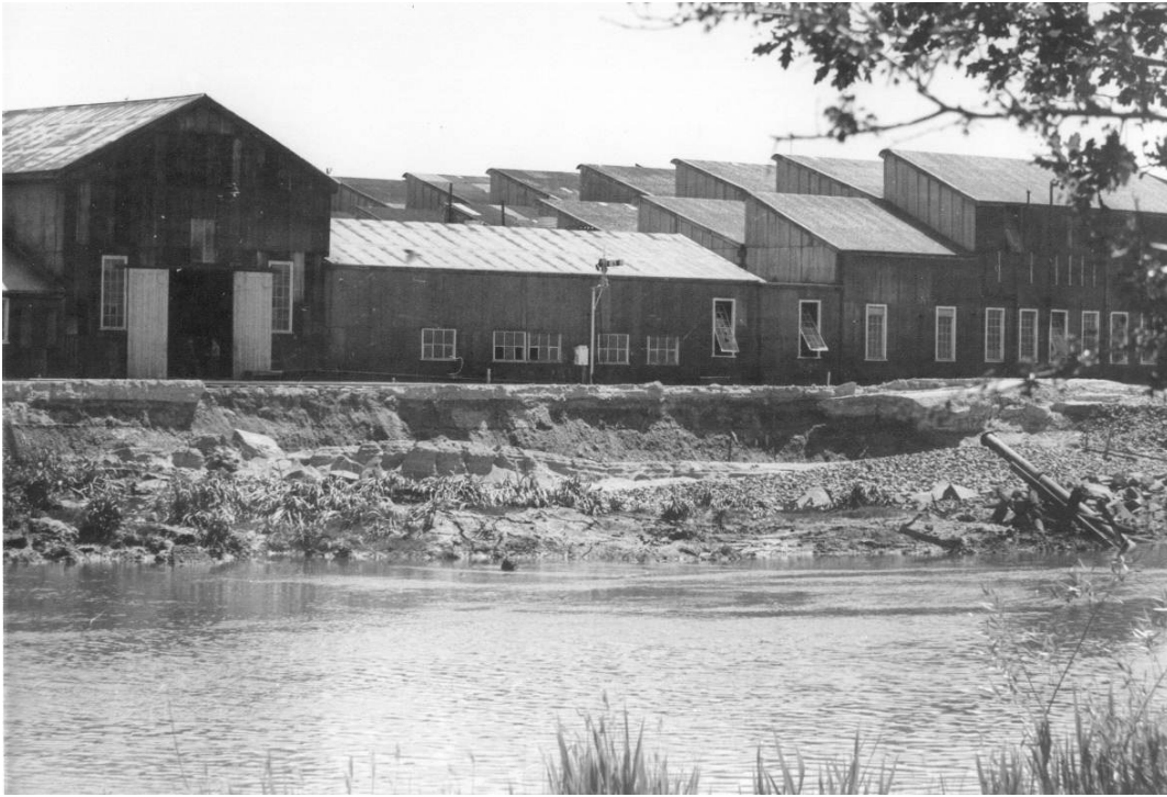
Figure 3 - Photo of the 1965 river bank slip at Invermay Railyards
