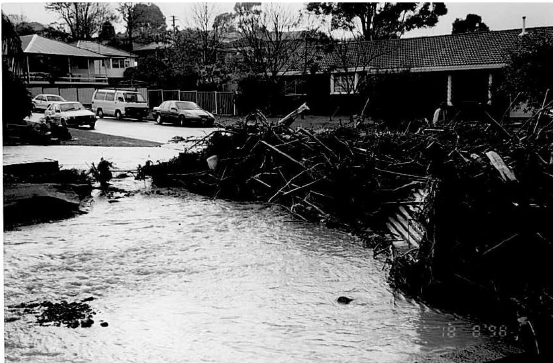
Figure 1: Blockage at Lemrac Avenue culvert in August 1998
